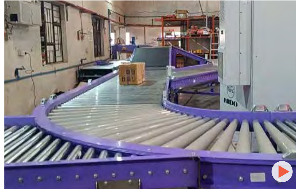
Conveyor automation | Conveyor automation with traffic management | Industry: Courier express parcel (Location: Bahrain)
