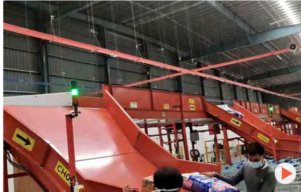
Volume distribution system | Conveying, sorting and volume distribution system | Industry: E-commerce
